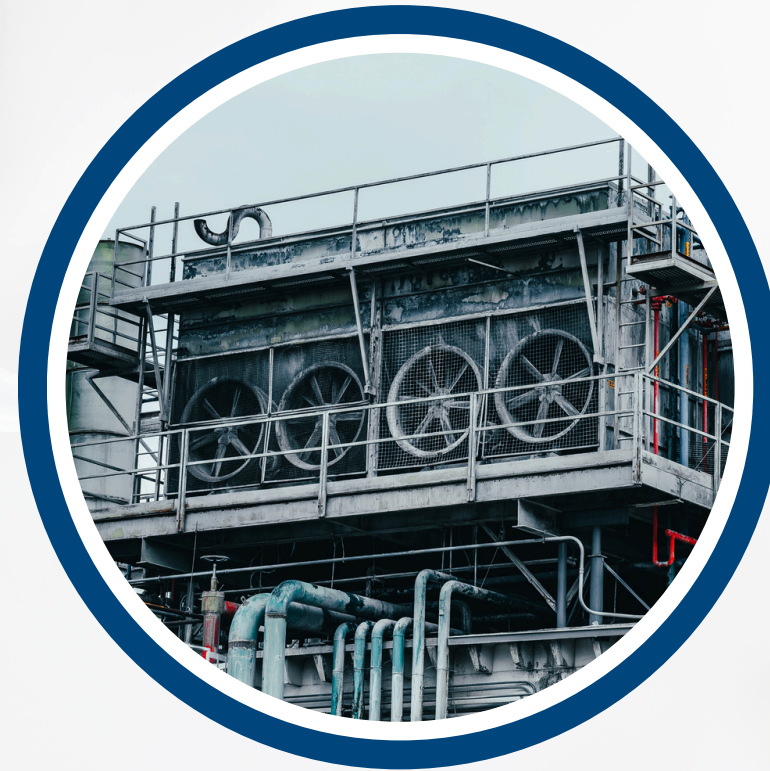
Liquid cooling & processing systems
